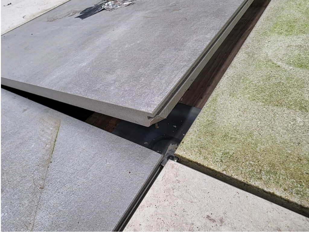
Plate 2 – Failure of Kerfed Edge at Wind Uplift Clip Location
