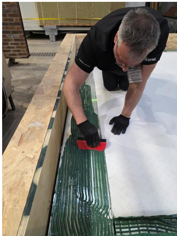
Plate 7 – Adhesive Installed Around the Perimeter of the Shockpad onto the Base Boards
